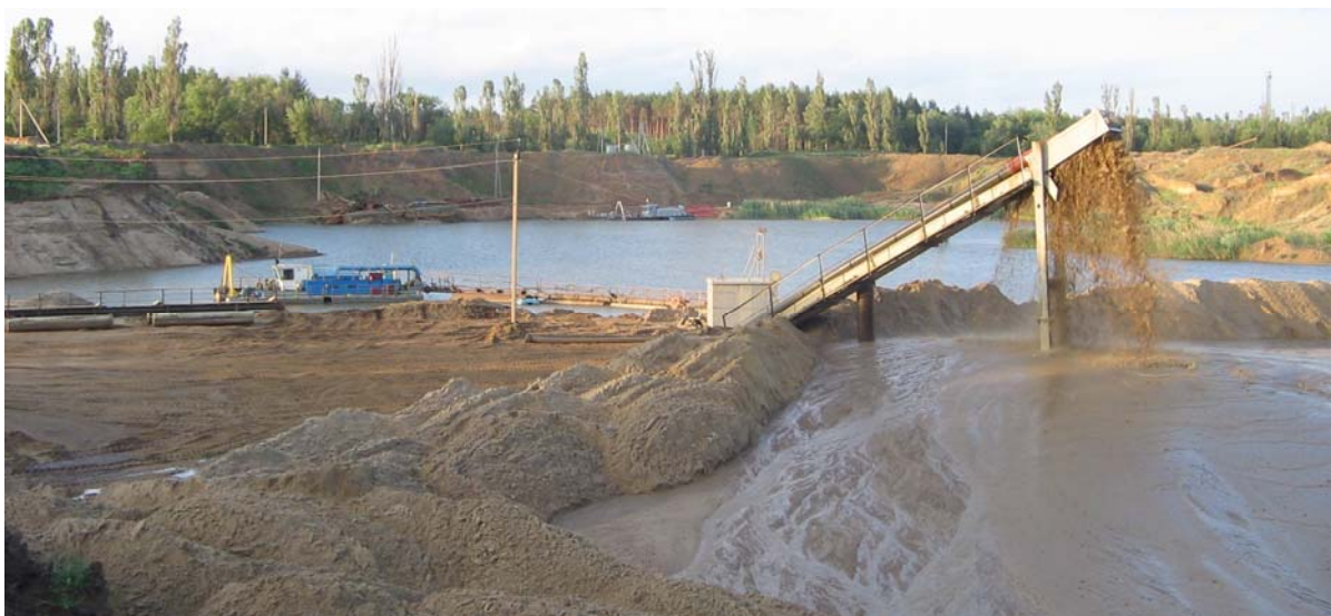
Fig. 2. Application of inclined screen GNK-1200
